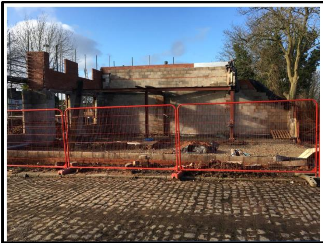
Photo 5 – looking west into site taken from Sunnybank showing extent of works commenced
